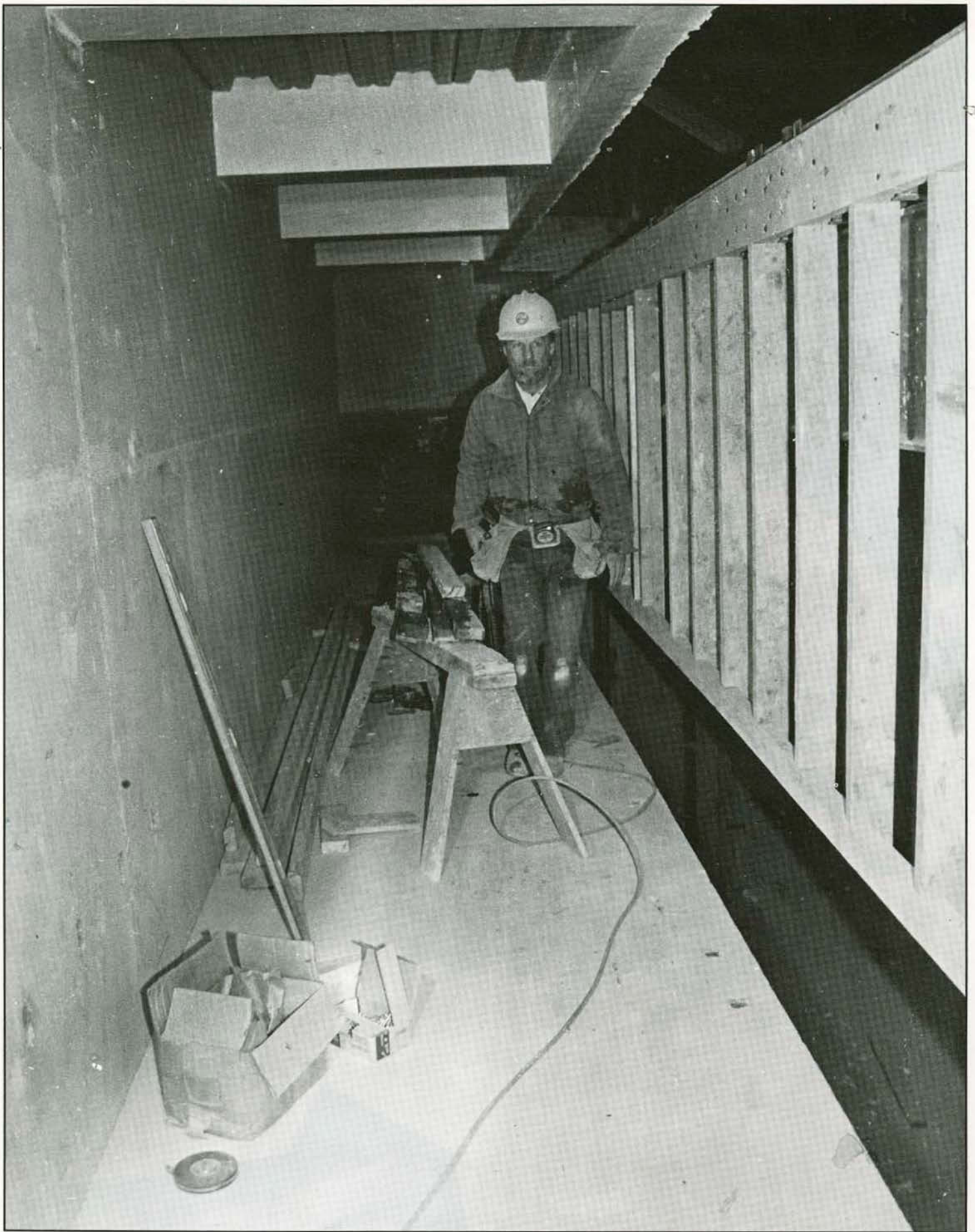
One of the many workers at Sheridan Coliseum examines the work that has been completed. By the end of the project, the building will have gone from a basketball court to a stage for a performance center. (Photo by Rene Kreutzer)
