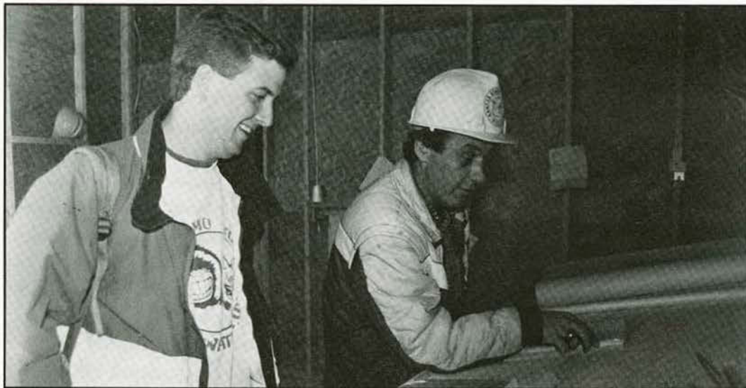
Tim Schmidt, Tulsa, Okla., junior, watches the construction foreman in Sheridan Coliseum.
