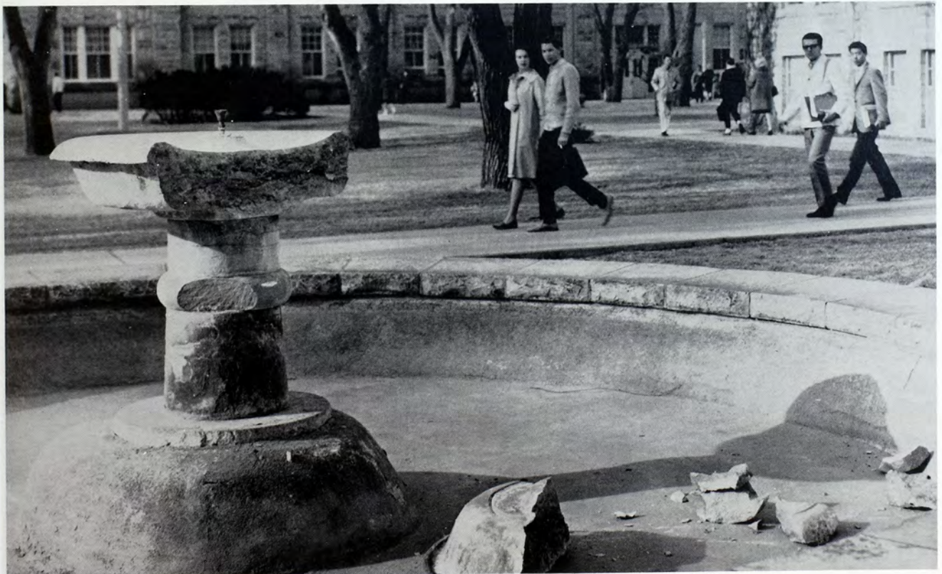
Passers-by observe breakage of the fountain, which was attributed to freezing and thawing.
