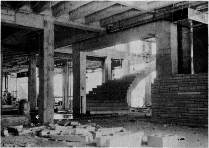
This is an interior view of the circular stairway in the Union as the building neared completion.
